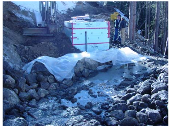
The vault for the pump equipment. This is now buried. The Creek water is flowing above the intake pipe.
