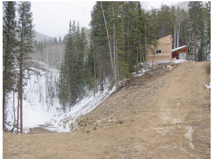
View of the status of the water repair work. On the left is the pipeline path to the Creek. The Creek intake area and pump vault is in the snow. The right side is the pipeline path to the new pump house. The existing pump house is behind the new one.
